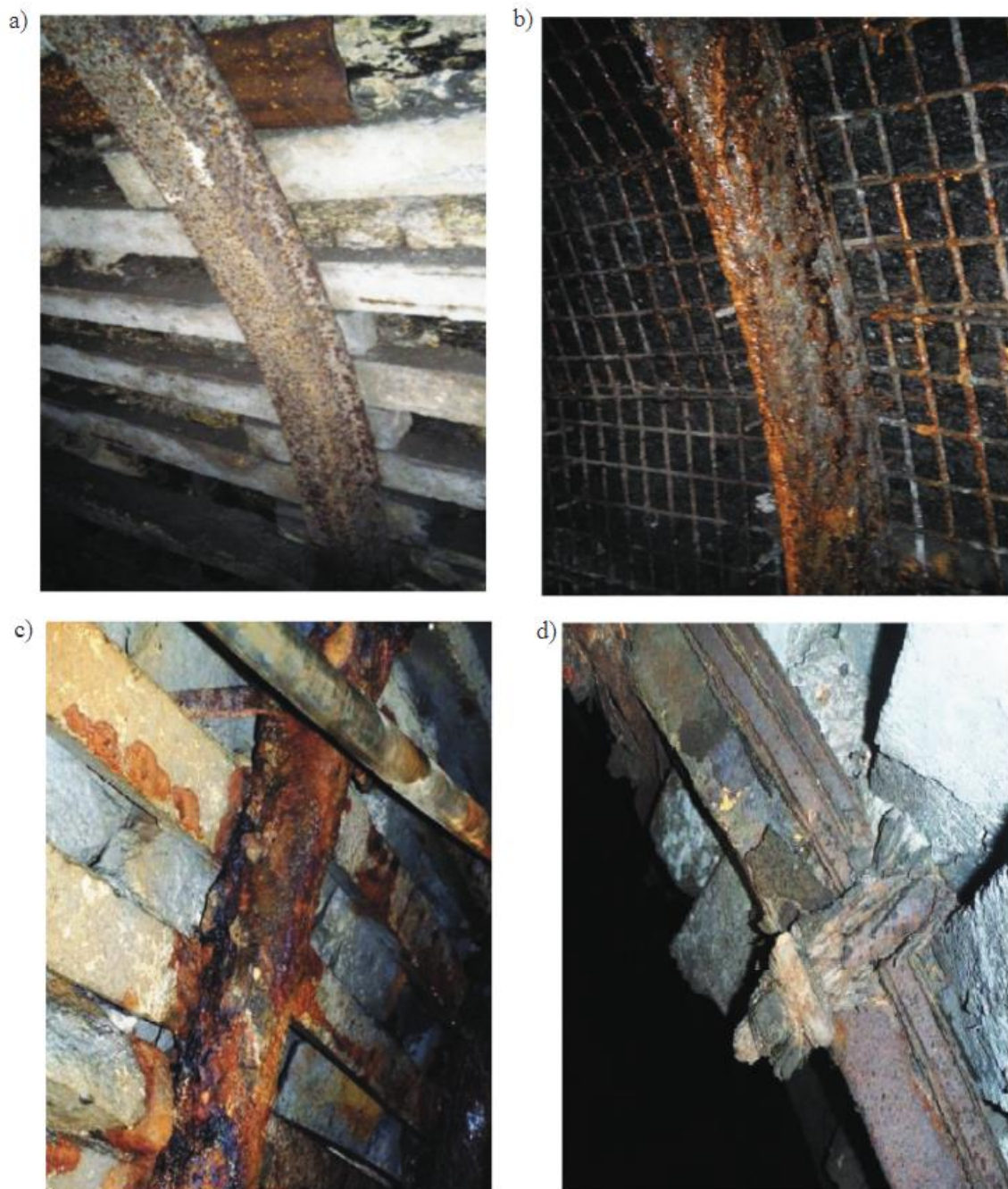
Fig. 3. Examples of steel arch support corrosion in Ziemowit part of Piast - Ziemowit coal mine: a - 1st level , northern crosscut, b – 2nd level, gallery 338, c – 3rd level, crosscut P-1, d - 3rd level, crosscut C-2.) (Rozmus & Ficek 2020)
