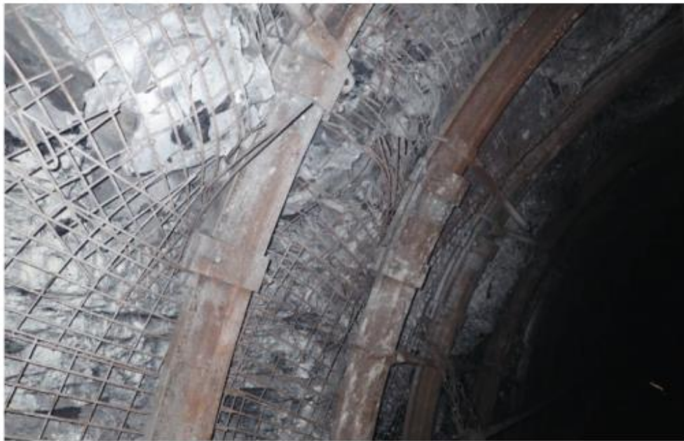
Fig. 5. The general view of main gate 25a – testing section I – only standing yielding support – the crushed coal in the sidewall with the left pillar (Małkowski and Niedbalski 2022)
