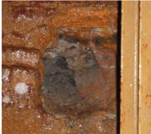
Figure 9 A notch in the shaft casing left by a girder
