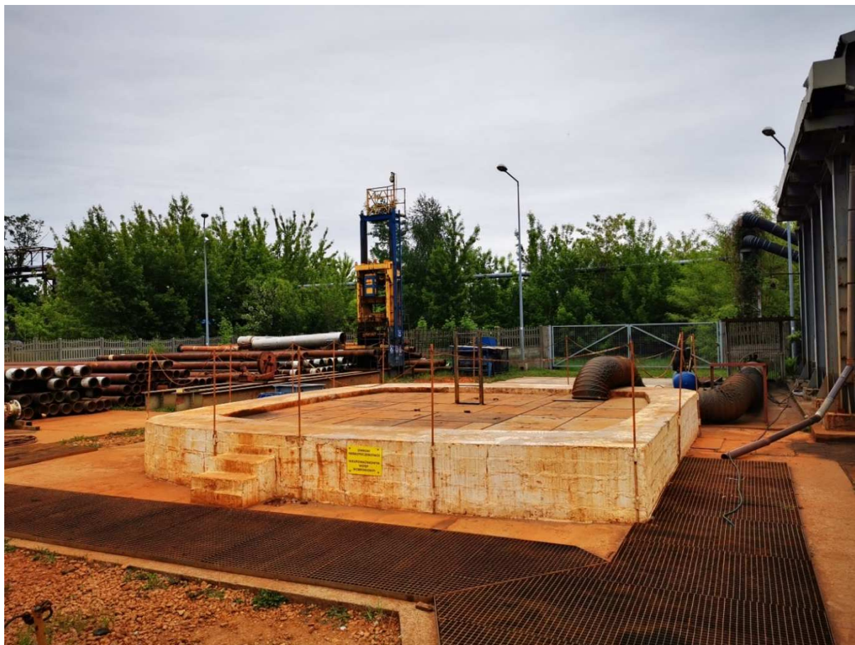
Fig. 38 PG "Saturn" - Bottom of the "Paweł" Shaft, at the back there is a device for lowering the pumps into the shaft [1]
