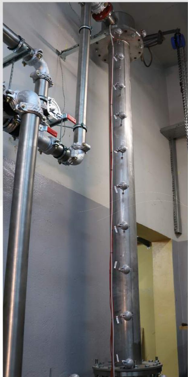
A TES tank without thermal insulation
