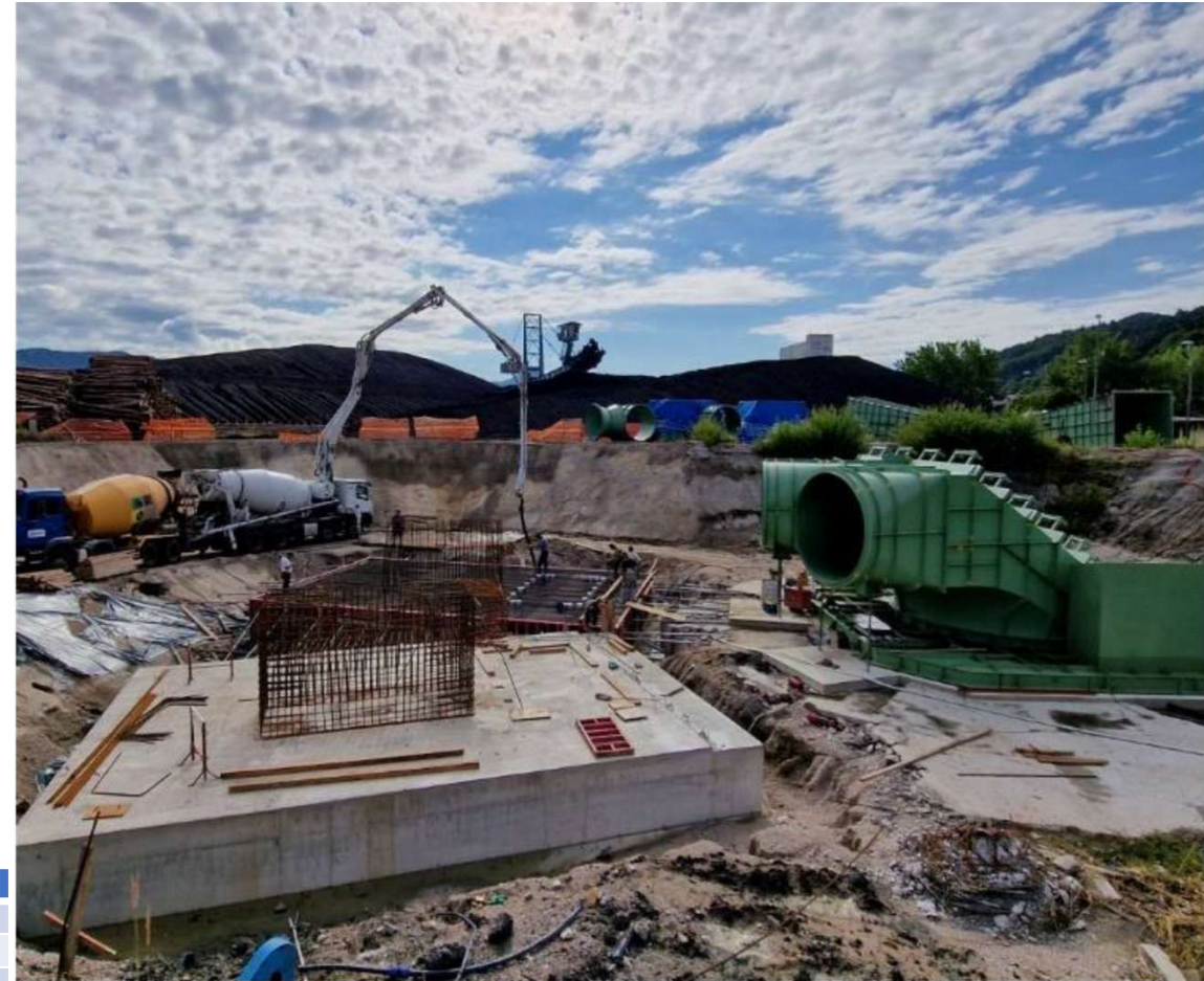
Fig 3: Ventilation Shaft Nove Preloge II – NOP II
