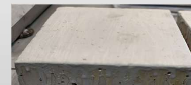
C20/25 + Sikagard WallCoat T after water erosion
